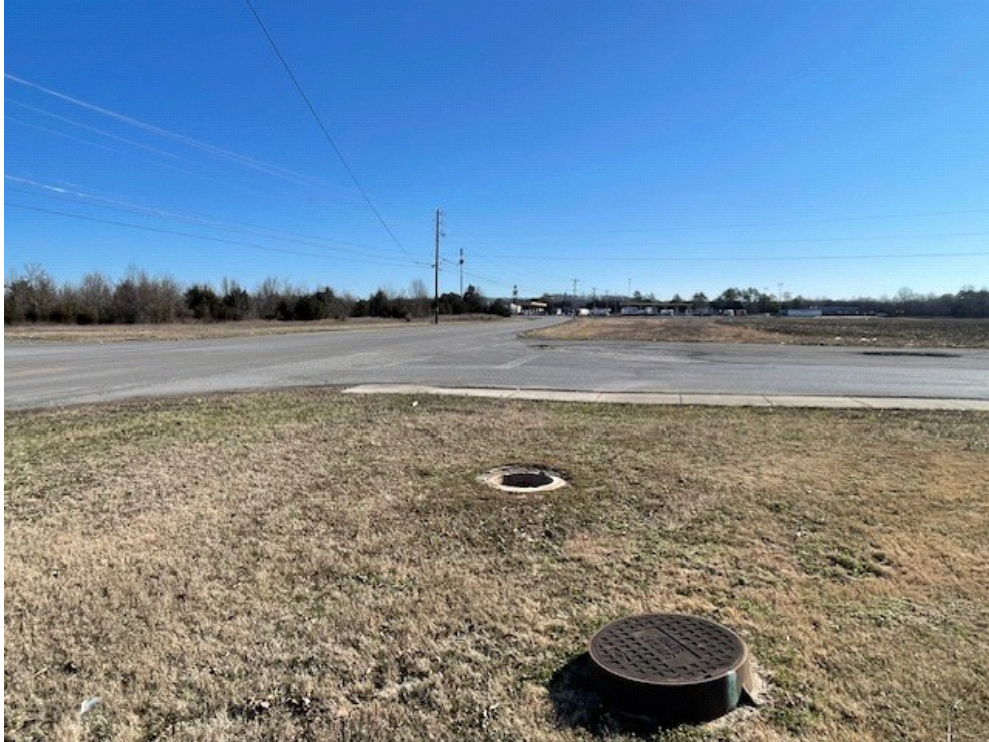
Sewer Manhole - Corner of Dollar General driveway facing east (one manhole, lid was off)
