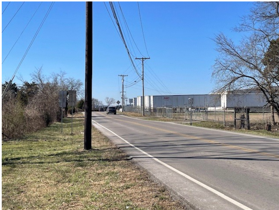
Power and AT&T Cable – Epps Mill Rd facing west near Manchester Pike
