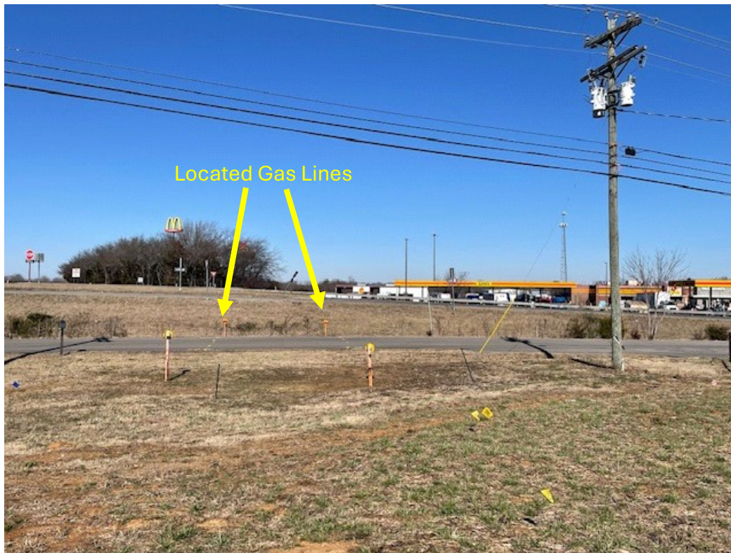
Gas Lines – Miller Ln facing north
